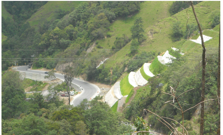
Treatment zone slopes of volcanic ash on shale formations. Slope terracing and a planted screens anchors in Manizales - Honda, PR 20 approx.
